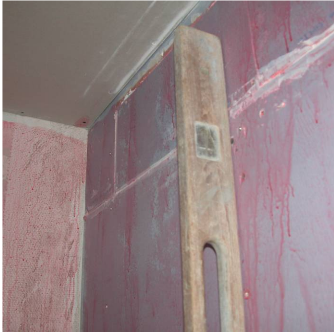
Photo 2: Unacceptable jump in level at the base for mounting of tiles
